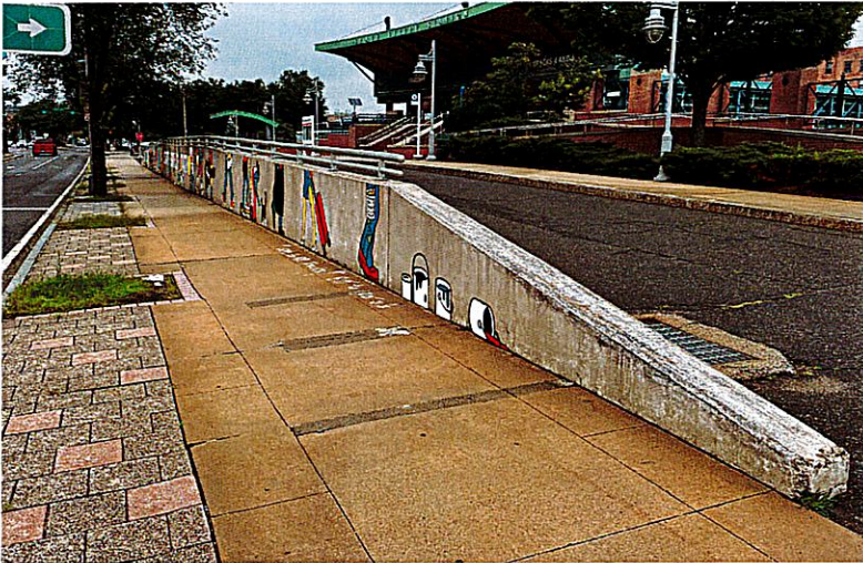
View of the wall from the sidewalk approaching the station from the south
